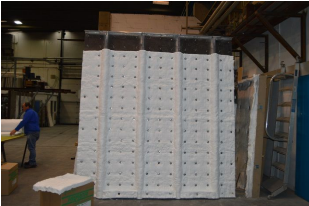
The aluminium bulkhead is getting insulated. Only one layer is used which is rolled over the stiffeners.
